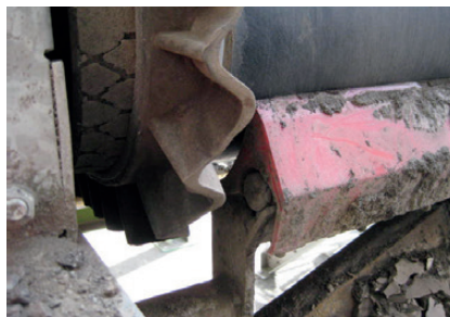
Cranked steel beam on corrugated sidewall belt
